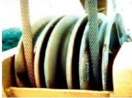
Inadequate inspection and maintenance
