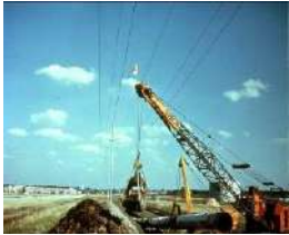
Working too close to power lines (minimum 10 feet)
