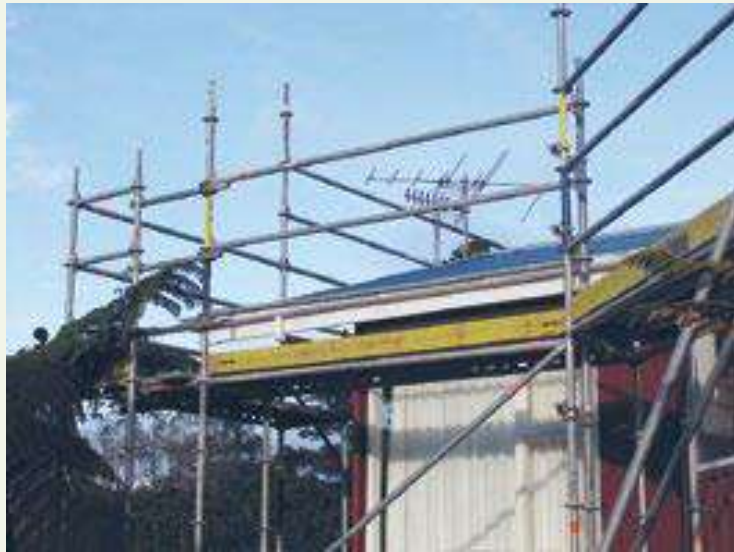
Example of edge protection on a roof of a residential home.
