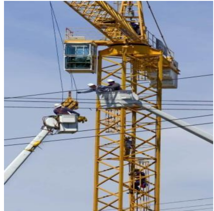
Crane hits Portland power lines; crane operator rescued
